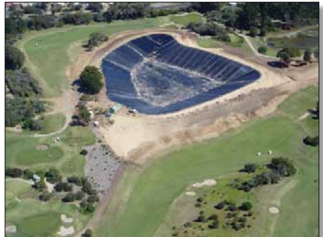
The Sam Wilson dam ready for storm water. We may never see the bottom again! We are still managing the vegetation works that we committed to during the planning and construction of this water storage.
